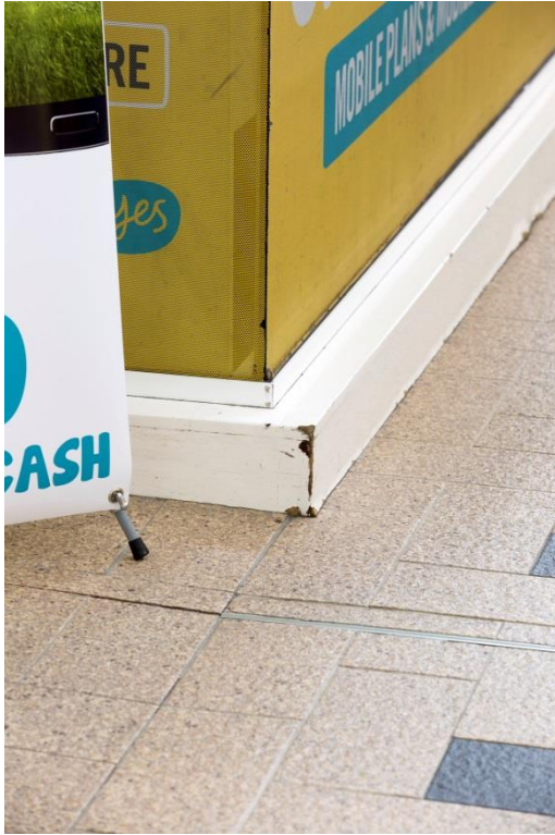
✗ Shopfront damage needs repair
