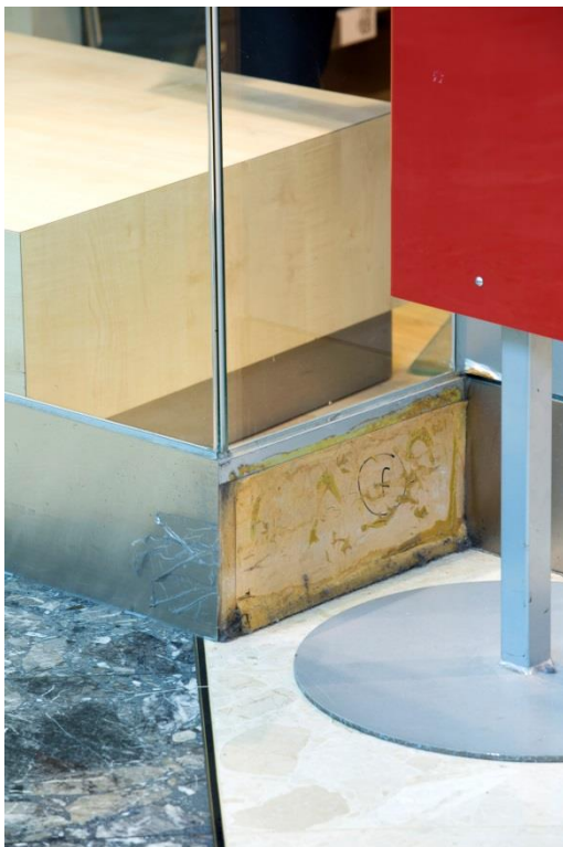
✗ Stainless trim missing
