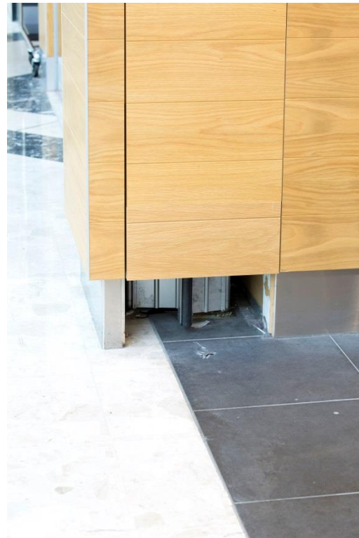
✗ Part of cupboard door missing
